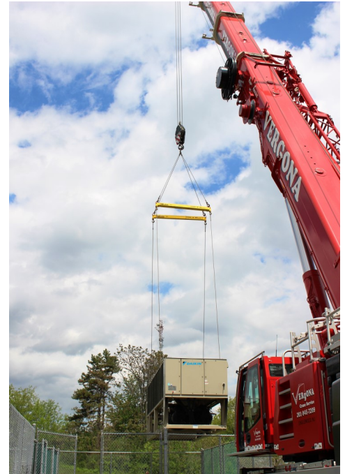
Vergona Crane Company (Englewood, NJ) rigging the new Daikin Pathfinder into place at Edison Municipal Building.
